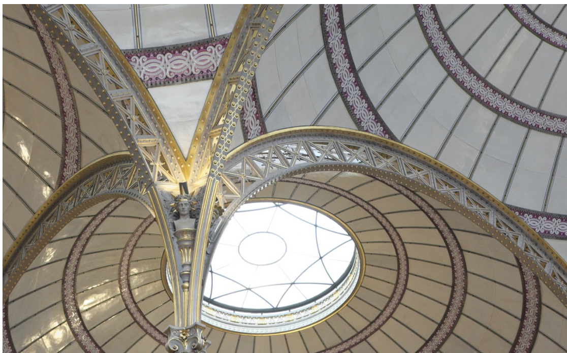
Figure 5. Close up of the cast iron arch roof beams of the Bibliotheque Nationale reading room
