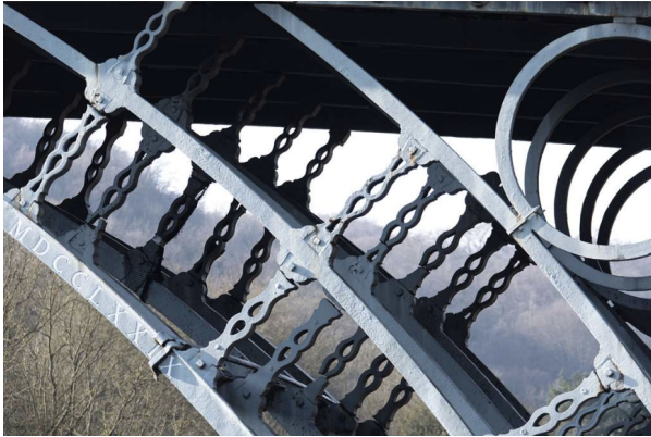
Figure 3: Details of the radial elements used on The Iron Bridge, showing the use of carpentry joints (English Heritage, 2020)
